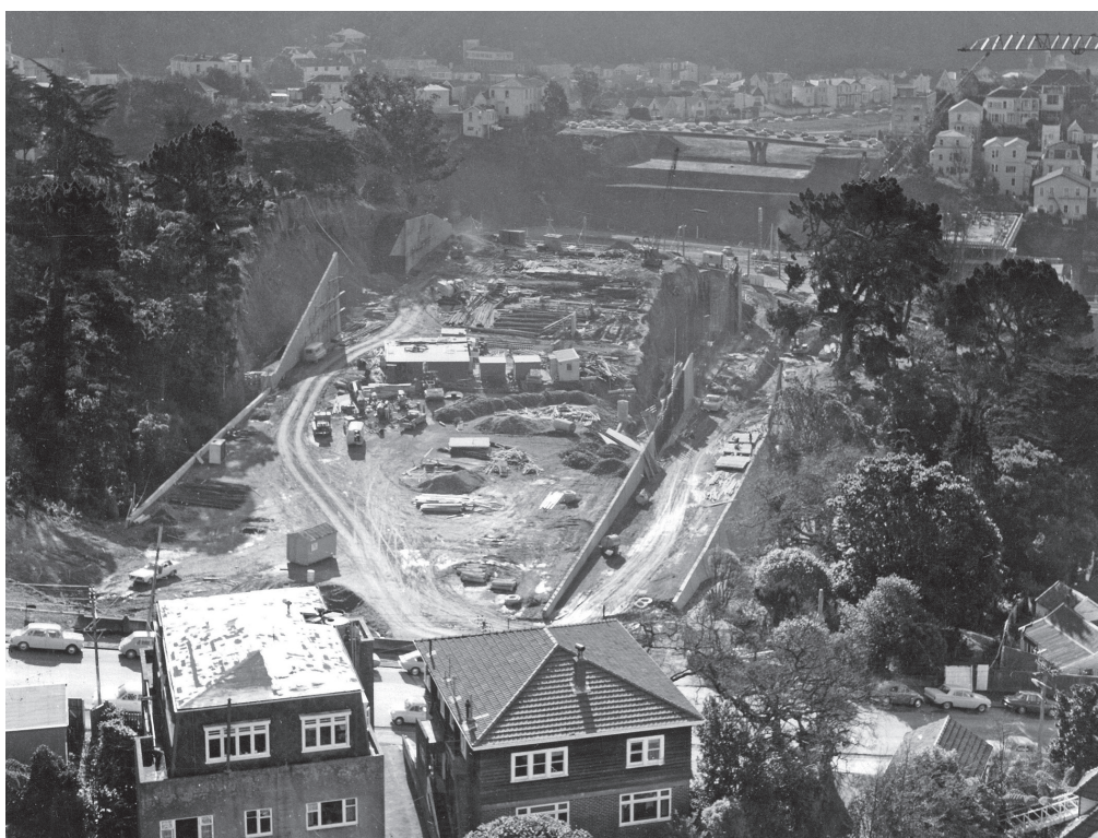
The main motorway trench being excavated through the former Bolton Street Cemetery, 1972.
